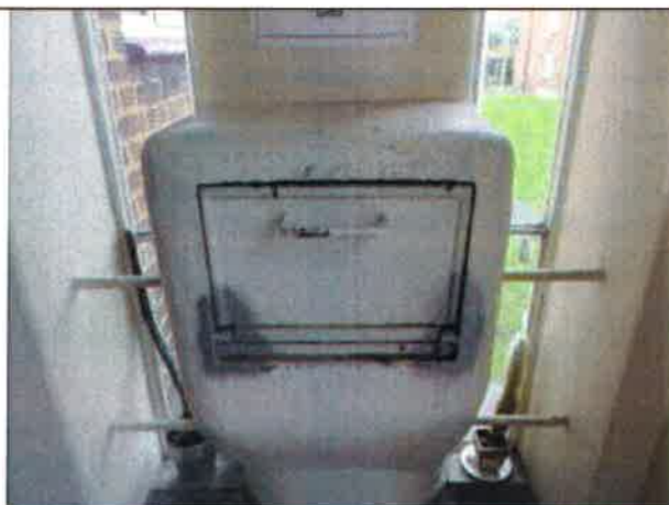
The refuse chute in the staircase enclosure
