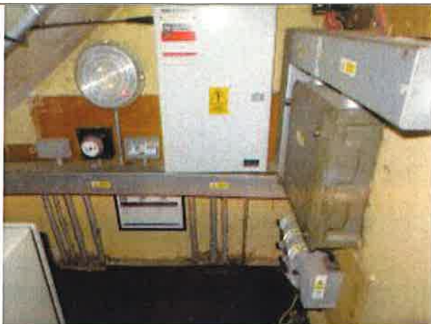
Inside electrical cupboard.
